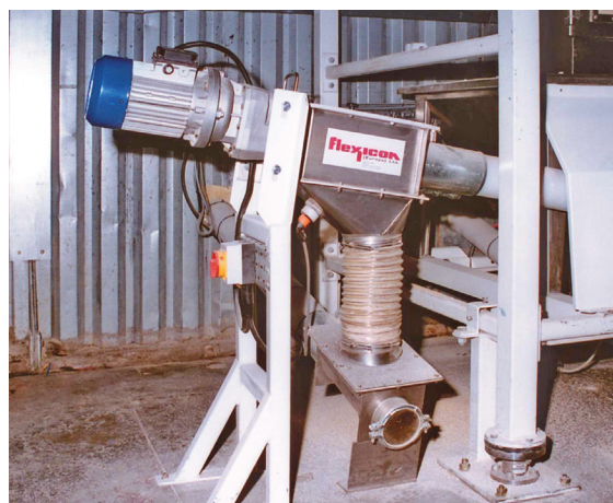
The flexible screw conveyors from both Bulk Discharge Handling Systems run parallel into the mixing station.
