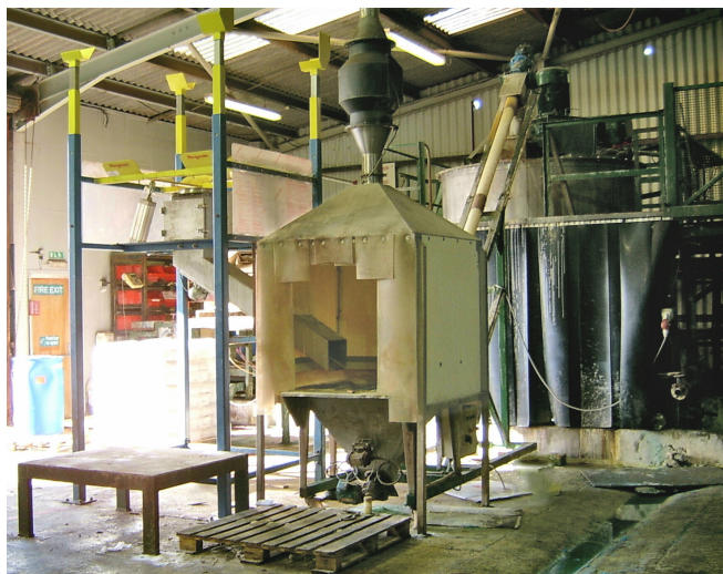
Bulk bag discharge system installed at Omex Agrifluids includes bag frame (upper left), FLOW-FLEXER® plates, hopper chute, and conveyor at rear that transports material to the blender.
