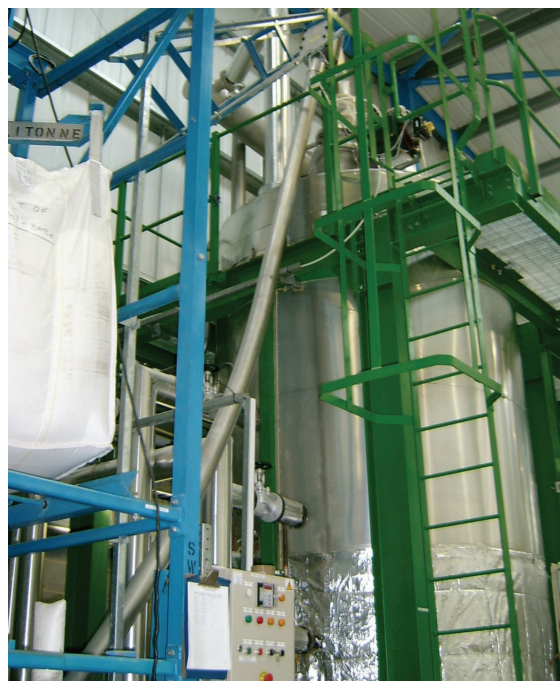
Flexible 6 m long (19.8 ft.) screw conveyor in polyethylene tube transports penta from hopper to the discharge-transition adapter, where it is gravity-fed into 5-tonne (11,020 lb.) reactor at M&I's Manchester UK plant.
