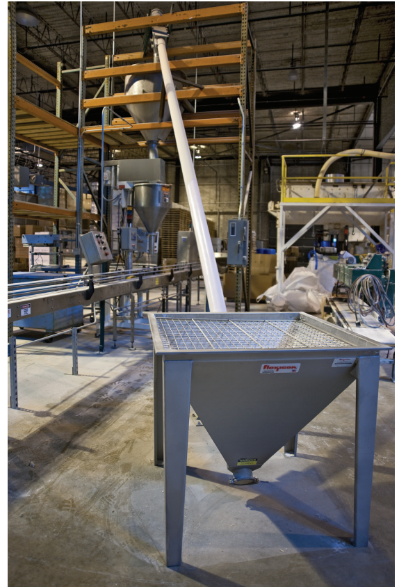
Blended perlite mixture discharges from bulk bag into the 8 cu ft (0.23 cu m) capacity stainless steel hopper (top), as the 30 ft (9.1 m) long flexible screw conveyor moves the material to the surge hopper above the packaging machine (above).
