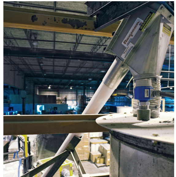
Material discharges from the conveyor tube through a transition adapter into the surge hopper.
