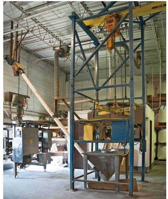
APCO Packaging employs bulk bag dischargers and flexible screw conveyors in repackaging various industrial, household and personal care products. This BULK-OUT® BFC discharger from Flexicon features a cantilevered I-beam with electric hoist and trolley.
